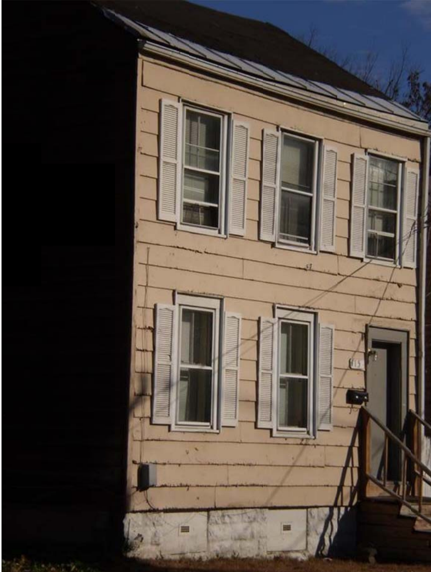
Figure 8: Minor Deterioration Example
